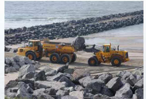
Large contractor's machinery has throughout the summer worked hard with the up to 24 tons heavy rocks.
